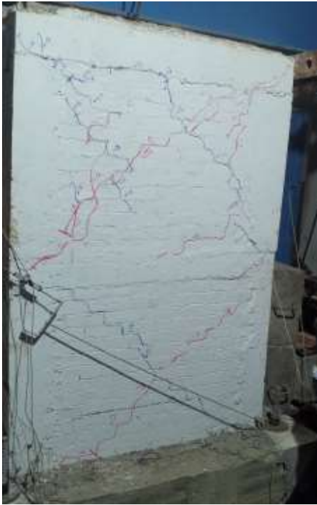
Fig. 13. DS6 Propagated Diagonal Shear cracks
