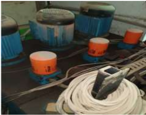
Fig. 6. Oil Hydraulic pumps used in testing.
